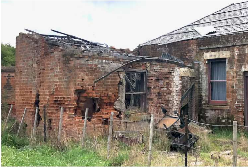
The former convict hospital doesn't have power or stormwater connections. (Supplied)
