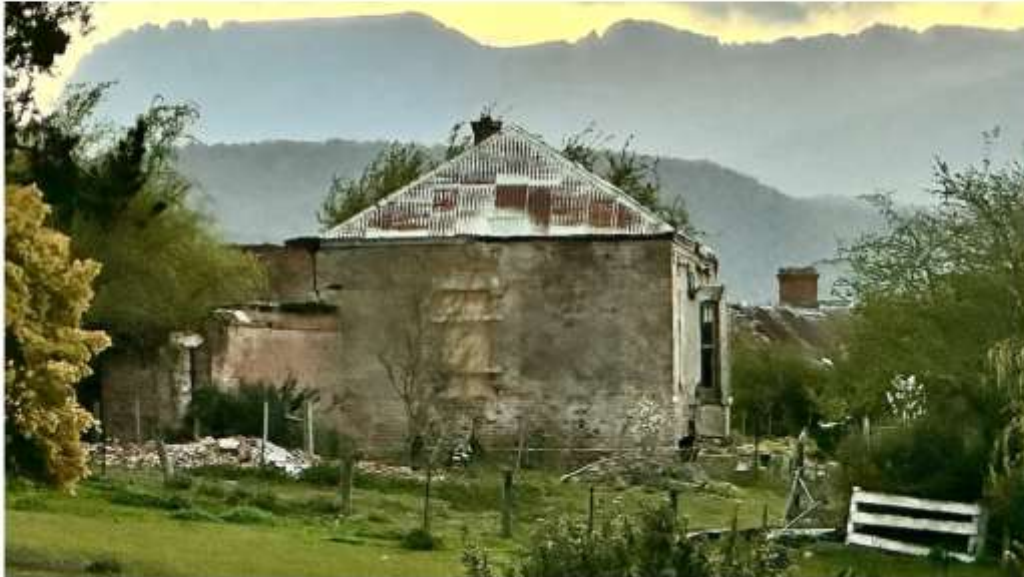
Set behind some houses, the crumbling remains of the 1840s convict hospital in Fingal, Tasmania, is easy to miss. (Supplied)
